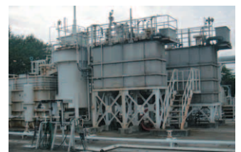
いわき工場水処理施設 Water treatment facilities in the Iwaki Plant
