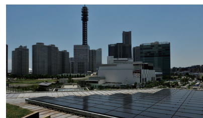
The solar panels installed at our Global Headquarters
