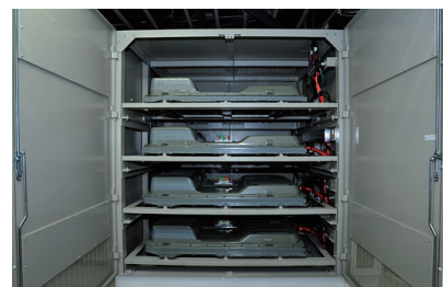
The energy storage system holds the equivalent of four Nissan LEAF batteries.
