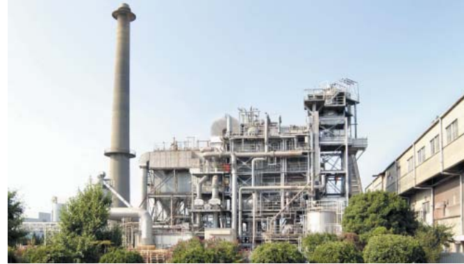
ASR recycling facility at the Oppama plant (Japan)
