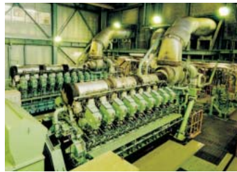
Cogeneration systems at Tochigi plant (Japan)
