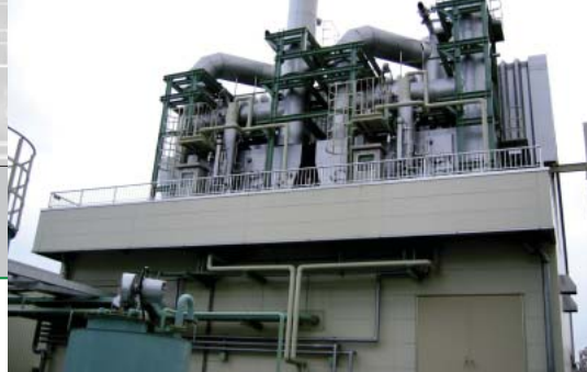
Installation of cogeneration systems using exhaust heat from power generation (Japan)
