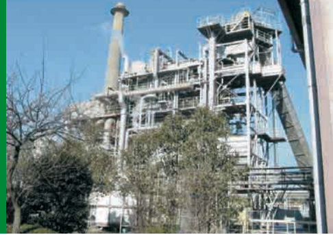
Equipment for the recovery of automobile shredder residue (Oppama plant, Japan)
