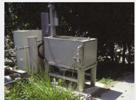
The device that automatically monitors rainwater quality
