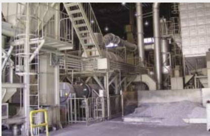
The aluminum sludge pre-processing furnace
