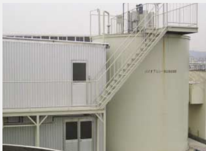
Heavy liquid waste processing facility
