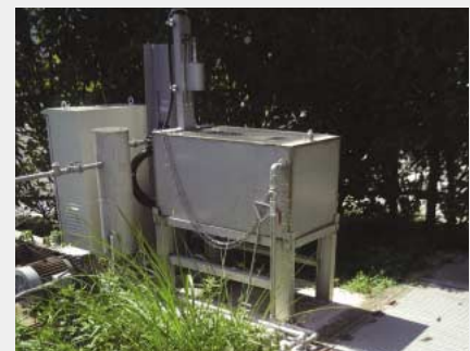
The device that automatically monitors rainwater quality
