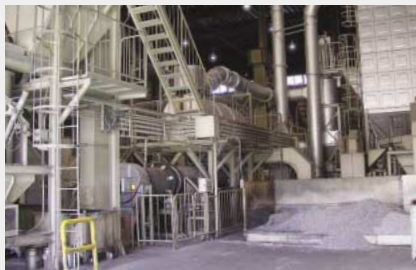
The aluminum sludge pre-processing furnace
