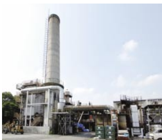
On-site incinerators in Tochigi Plant
