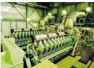
Cogeneration system in Tochigi Plant
