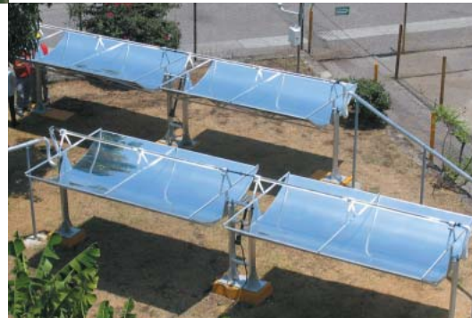
Using solar-powered hot water for employees' shower (Aguascalientes Plant, Mexico)
