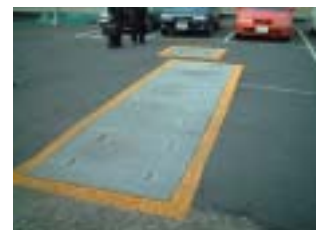
Yellow display to aid identification of oil-separation equipment positions
